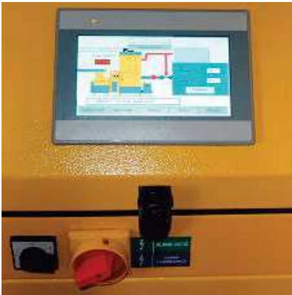
Main switch and control panel
