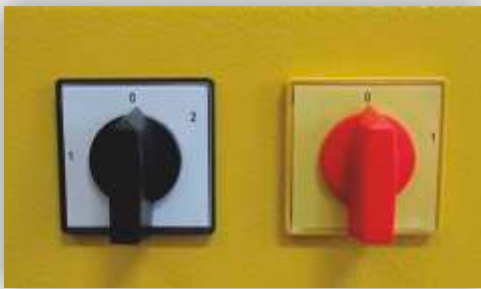
Main switch panel
