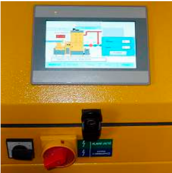
Main switch and control panel
